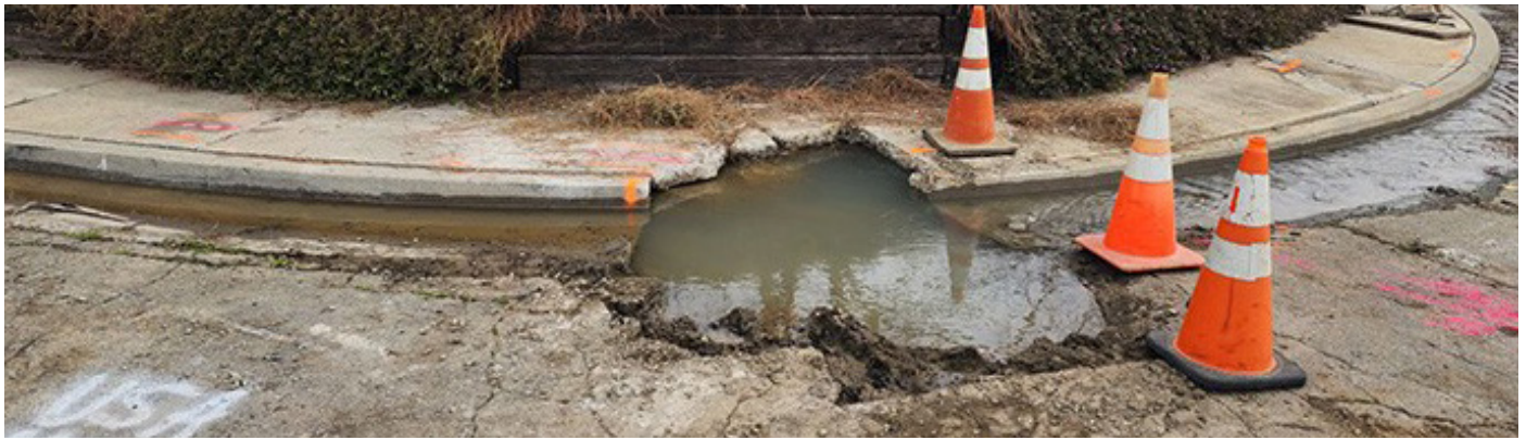
Damage caused by failing infrastructure in Madison. Photo credit: Yolo Subbasin Groundwater Agency staff.
